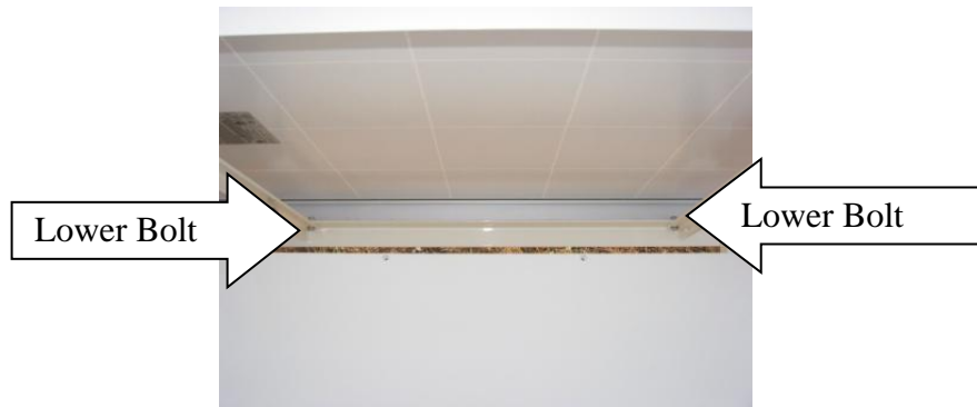
Figure 9. Lower Solar Panel Mounting Bolts
